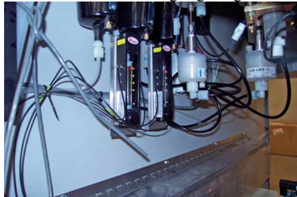
Flow meters with photo-eyes verify the coating pumps are working. Past the flow meters are the pumps. They are mounted on the back wall of the under deck area.
